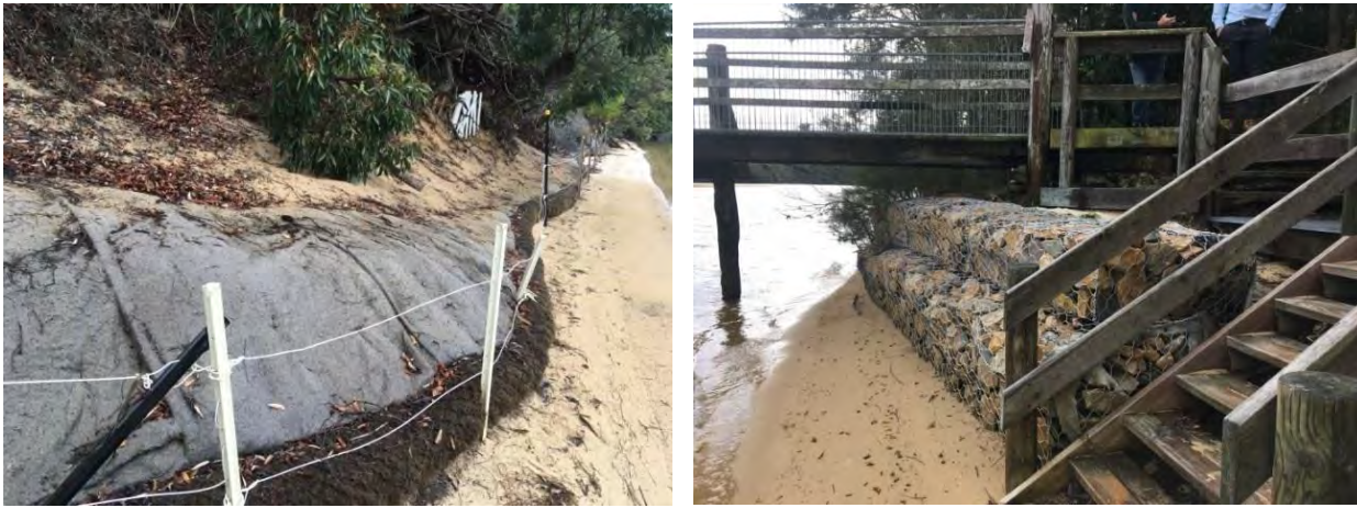
Plate 20: Left: Appropriate treatment of unconsolidated banks using geofabric and coir log combination, Warrell Creek (July 2018); Right: Rock gabions used to remediate bank erosion under Deep Creek footbridge (July 2018)
