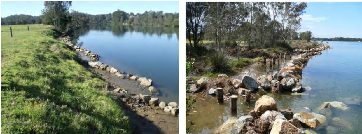
Plate 21: Left: Bank stabilisation at Wirrimbi (2017); Right: Recycled stumps used in bank stabilisation works (Landcare, 2019)
