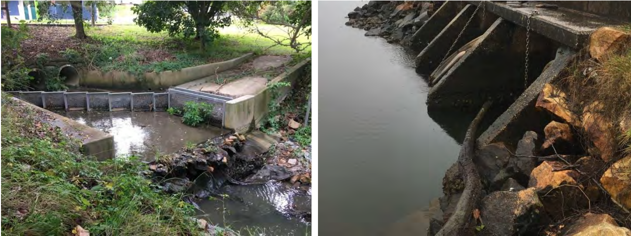
Figure 9: Left: Gross Pollutant Trap at Bellwood Park; Right: damaged floodgate at East Street, Macksville (July 2018)
