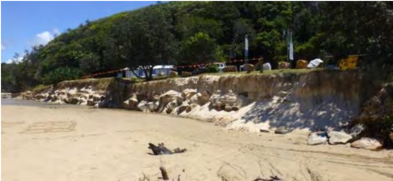
Plate 16: Poor design of seawall at South Valla Beach car park (February 2018)
