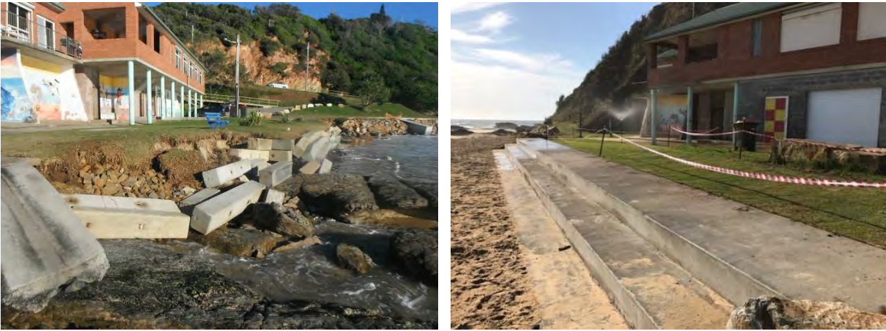
Plate 12: Left: Nambucca Main Beach Surf Club access stairs damaged by storm events; Right: Main Beach Surf Club after replacement of access stairs
