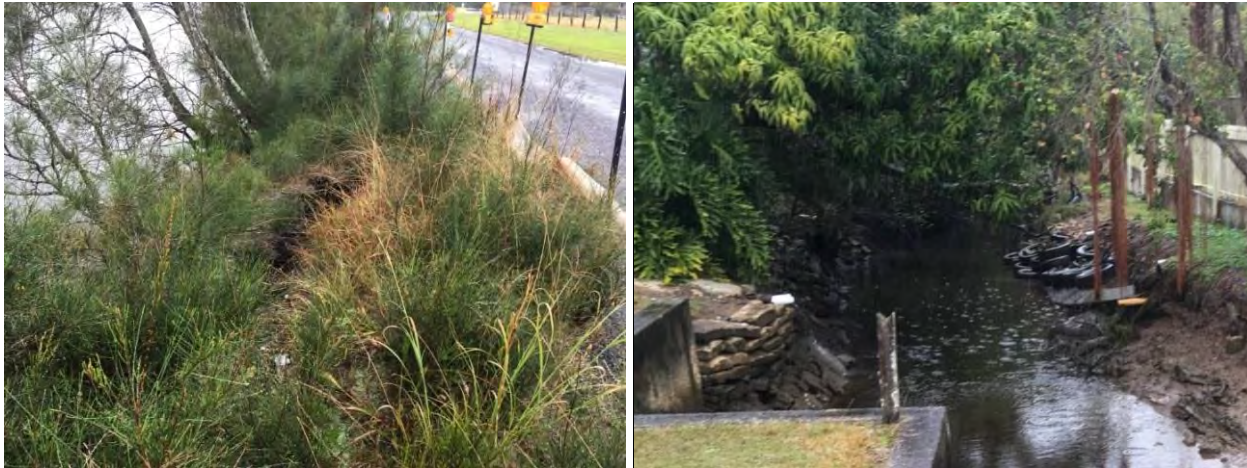
Plate 19: Left: Slumping of the bank adjacent to Gumma Road (July 2018); Right: Unlicensed foreshore protection structures, Macksville (July 2018)
