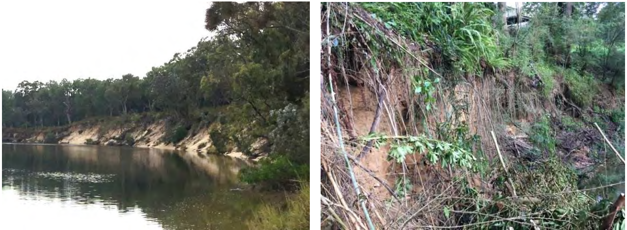
Plate 18: Left: Unstable unconsolidated sand banks in Warrell Creek (July, 2018); Right: Severe bank instability and undercutting on the South Arm, upstream of Bowraville (July, 2018)
